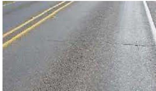
Gambar 2. 8. Retak melintang ( vertical cracks )
